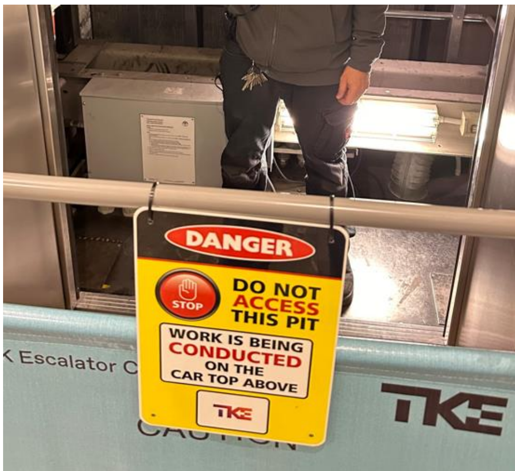
Lower Level / Pit Danger Signage
