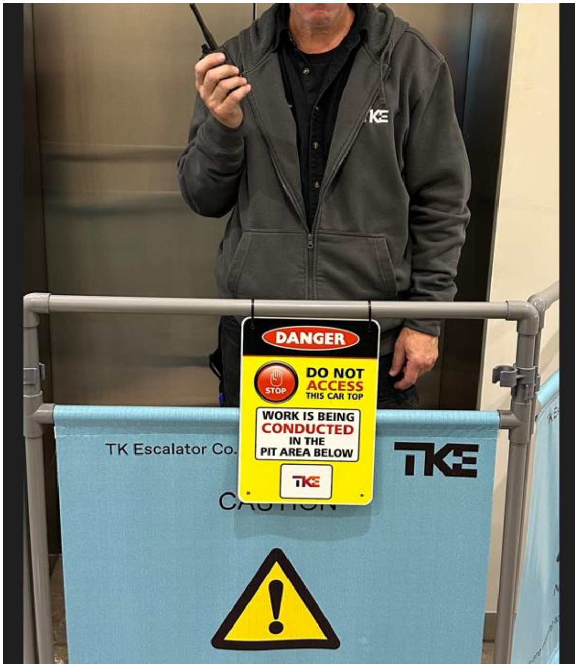
Upper Level / Car Top Danger Signage
